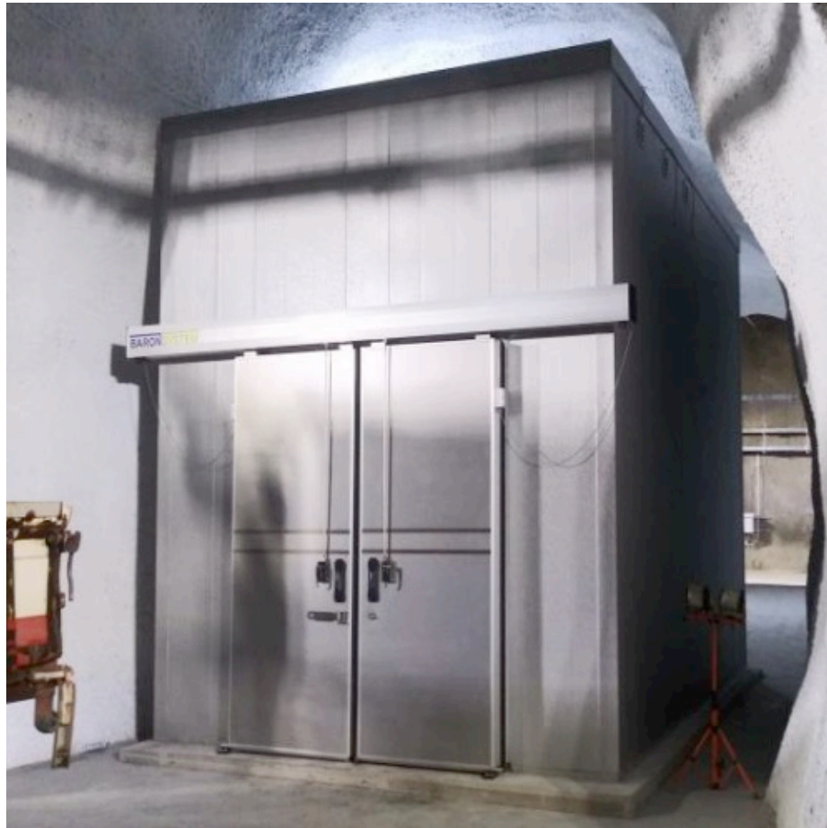
Freeze room for -30°C operation
